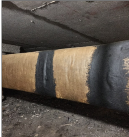
Photograph No. 24: Asbestos-containing black tar mastic on ducting within the south crawlspace (Samples 0007A-C).
