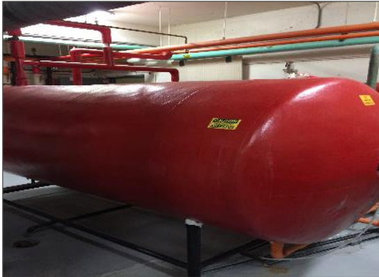
Photograph No. 3: Asbestos-containing parging cement present as insulation on the hot water holding tanks within the pool room Loc.13.
