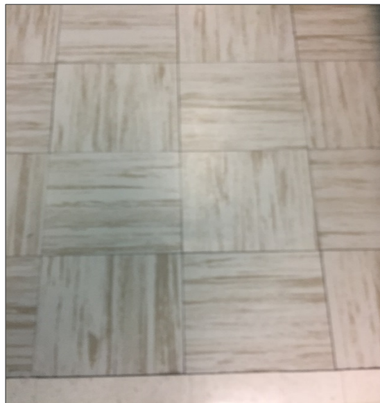
Photograph No. 13: Asbestos-containing vinyl floor tiles within pool corridor and office Loc.'s 38 and 43 (Samples 0033A-C).
