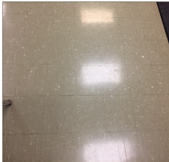
Photograph No. 15: Asbestos-containing vinyl floor tiles within the cloak room Loc.47 (Samples 0038A-C).
