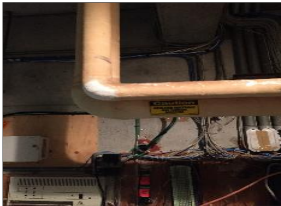
Photograph No. 1: Asbestos-containing parging cement present on fittings, elbows, valves and tee's of the Domestic, hot water, steam system.
