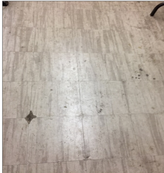
Photograph No. 12: Asbestos-containing vinyl floor tiles within the rink sound room Loc.15 (Samples 0023A-C).
