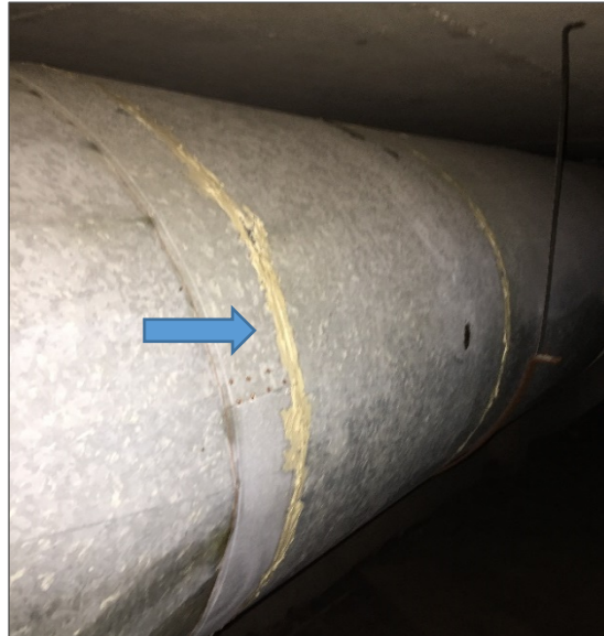
Photograph No. 26: Asbestos-containing beige mastic present on uninsulated ducting within the south crawlspace and basement board room (Samples 0008A-C).
