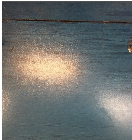
Photograph No. : Non-asbestos blue matting within the Reception area and Gym Loc.'s 30 and 42 (Samples 0030A-C).
