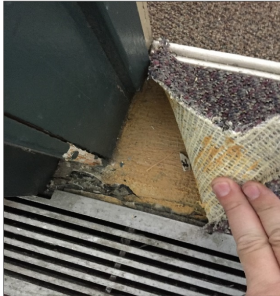
Photograph No. 20: Asbestos-containing vinyl floor tiles within the mezzanine board room and storage room under carpeting Loc.'s 66 and 67 (Samples 0053A-C).
